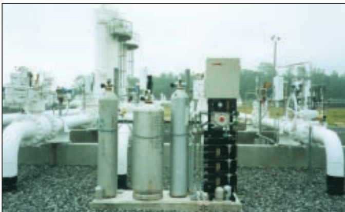
Typical outdoor installation in U.S. Gulf Coast region.
